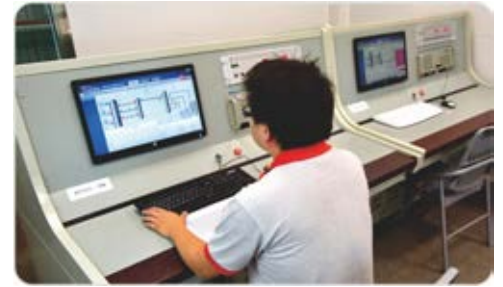
Control room & Graphical HMI
