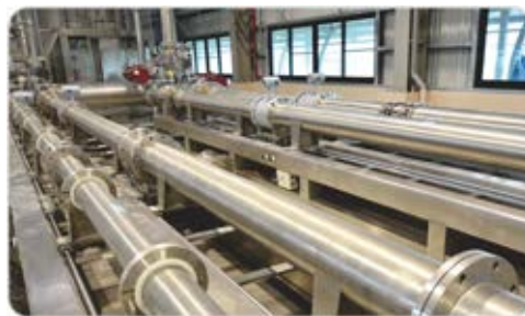
Piping system II (Maximum diameter is 300mm)
