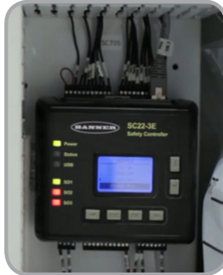
SC22-3E Safety Controller installed in the Universal-8 Packaging System
